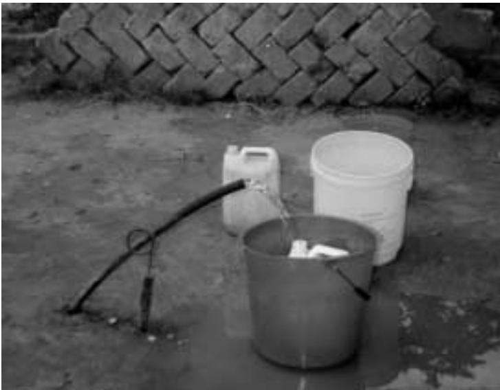
Drawing water from a damaged pipeline in Temeke
