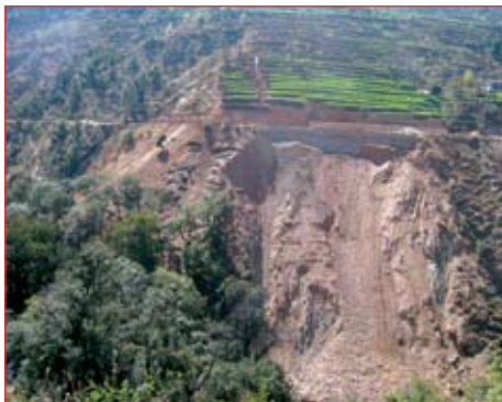
Land degradation – disturbed slope due to road construction (Bajhang District)
