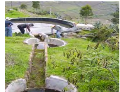
From road runoff
