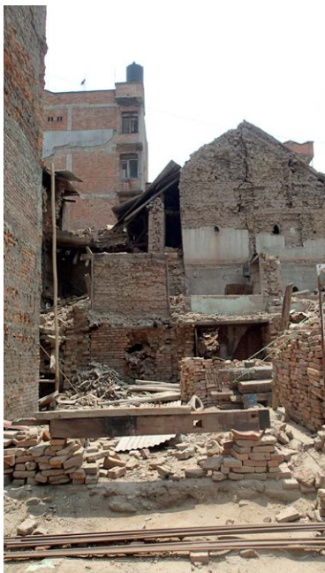
5a: Demolished building with rubble piled up, Pilachhen.
