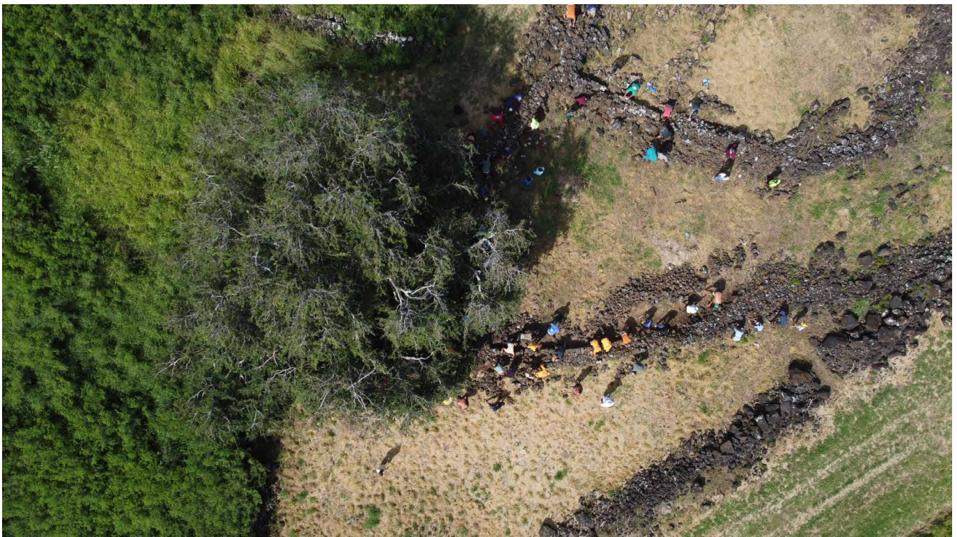
Fortifying the wall foundation at Hô'ai, Kaua'i at the Hui Malama Loko I'a Gathering 2023
