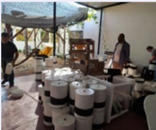
Installing the chambers in a livestock farm in the municipality of Paz de Ariporo (Casanare) Credit: Héctor William Moreno Quitián
