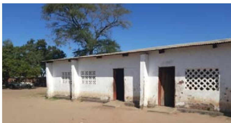
Figure 2. One of the school blocks at Mitole Primary School, which is also used as a disaster shelter. Credit: Chancy Sibakwe
