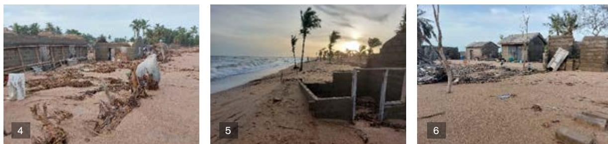
Figures 4, 5 and 6. Households destroyed (4), buried in sea sands above window level (5) and abandoned by occupants (6) after tidal waves at Agorkedzi. Credit: Sylvanus S.P. Doe
